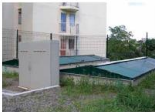
Plateau Tiberge (Martinique), 400 PE, Ecodisk installed right next to homes
